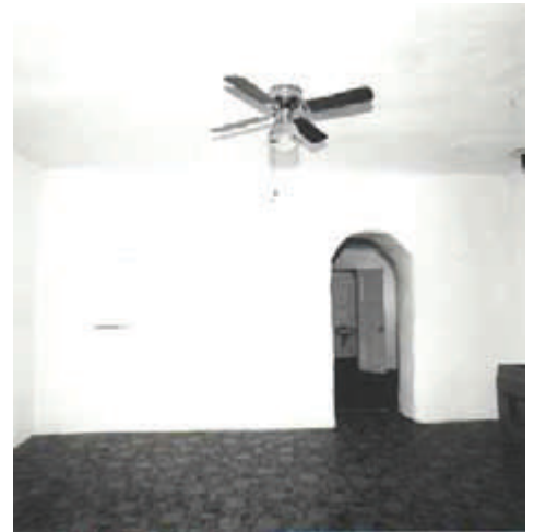
The Garcia House, north room, before the restoration. The oak floor was beneath linoleum. Photo by Hope Curtis.
