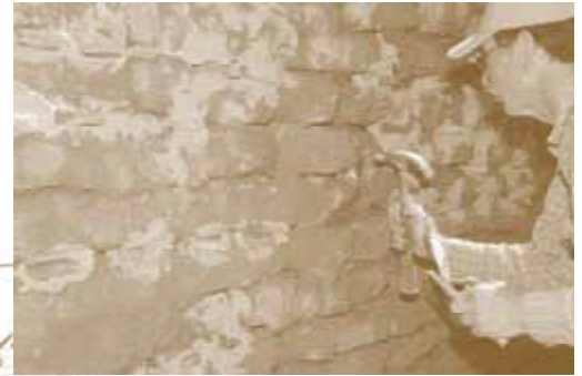
Charles Coffman installs stones set in lime which act as a key system to hold the lime plaster on the entrance wall at El Zaguán.
