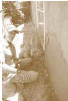
Right the Donaciano Vigil House received a fresh coat of mud plaster this summer. The work also included the installation of a drainage system to protect the foundation.
