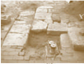
Left, these things always seem to happen in the dead of winter. Rebuilding a drain line at the Vigil House was one of our first projects of the year.
